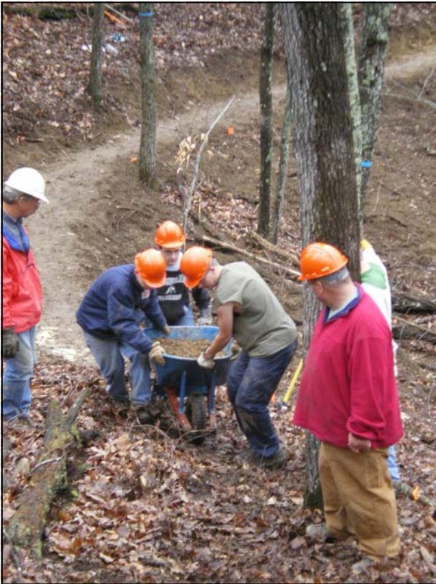
Caleb Wilson, John Wells, and Zack Whitehead bring up a load of dirt up the newly installed Bee Creek Trail at Latimer High Adventure Reservation.
